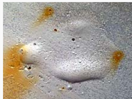
BLEED THROUGH AFTER AN IMPROPER REPAIR
